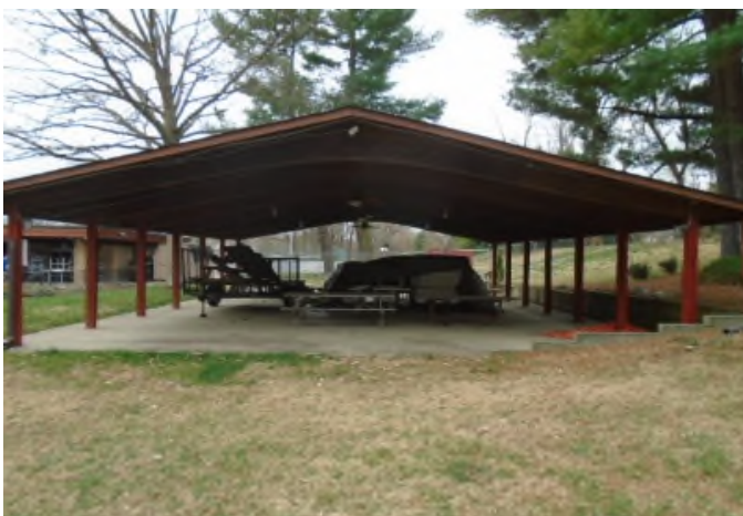
Pavilion structure is considered a "life of the property" component. Reserves provide for replacement of shingle roof, gutters/downspouts, concrete repairs, light fixtures, and ceiling fans.
