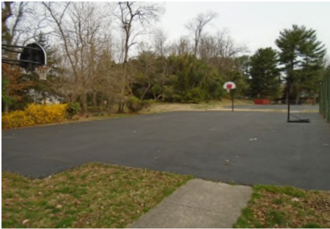
Basketball ball court without markings requires periodic crack filling and sealcoating. Mill and overlay will be required at end of useful life.
