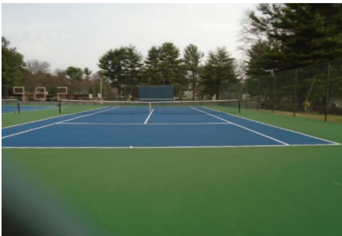
Tennis/pickleball courts were renovated in 2021. Reserves provide for periodic crack sealing and color coating. Major repairs are needed when cracks and surface areas deteriorate.
