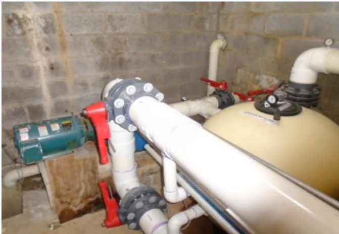
Reserve provides for pool filters, water supply/return piping, chemical equipment and other system components.
