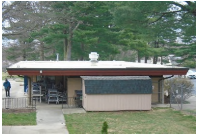
Side view of building showing flat roof with single ply membrane roof. Roof has had minor repairs and is reportedly not leaking. Reserves provide for replacement when needed.
