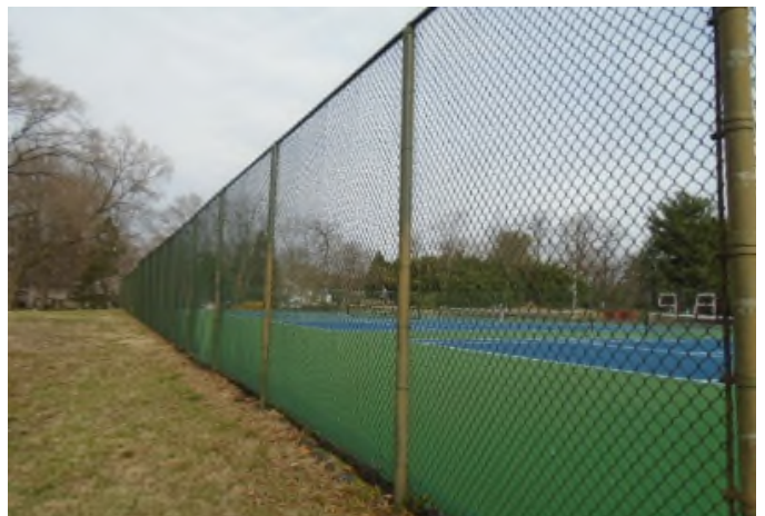
Chain link fence at tennis/pickleball courts useful life can be extended by replacing missing tie wires, stretching fabric and painting to control rust.
