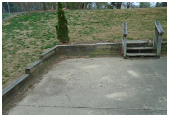
Replacement of wood retaining wall and steps at the pavilion are included in the reserves.
