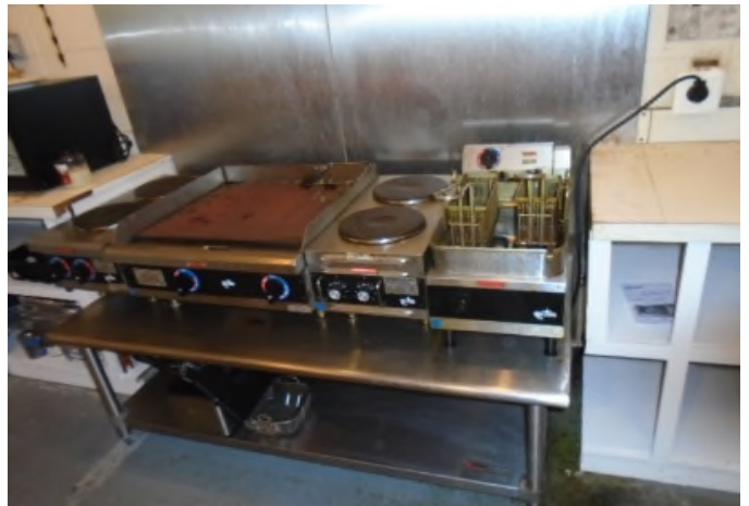
Snack bar is a leased space. Equipment is the responsibility of the operator and is excluded from the reserves.
